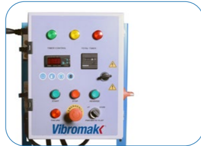
Electric Control Panel Elektrik Panosu
